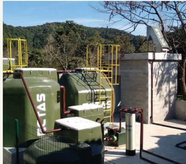
Customised solutions reduce the cost of sewage treatment
